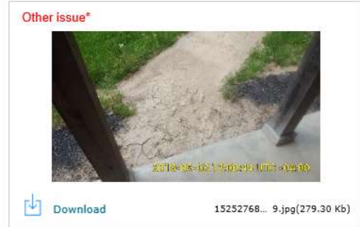
Sidewalk covered in mud
