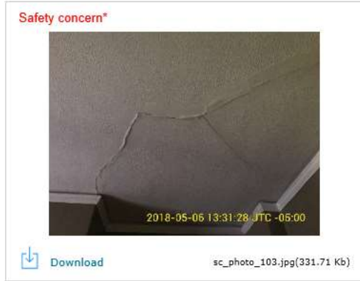
Crack in ceiling
